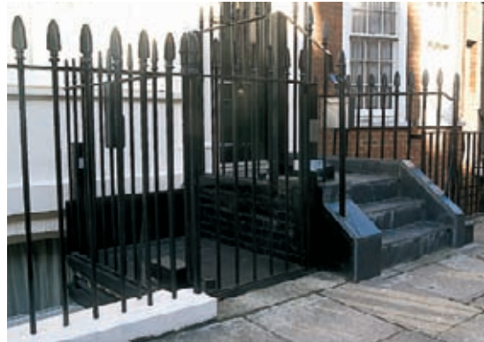
Many entrances to 18th-century and 19th-century terraced town houses have steps up to the front entrance, along with a basement area. An external platform lift was installed within the basement area of this London house, the steps and landing altered and the railings adapted in keeping with the existing design. A lift was installed within the house. The house has since been sold and the platform lift removed.
